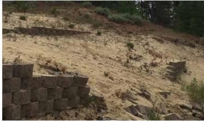
Prior to the project, this sandy embankment contributed significant amounts of sediment to Lake Cascade.
